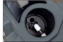
Reliable 120V Transfer Pump capable of transferring 30 GPM of water to the holding tank
